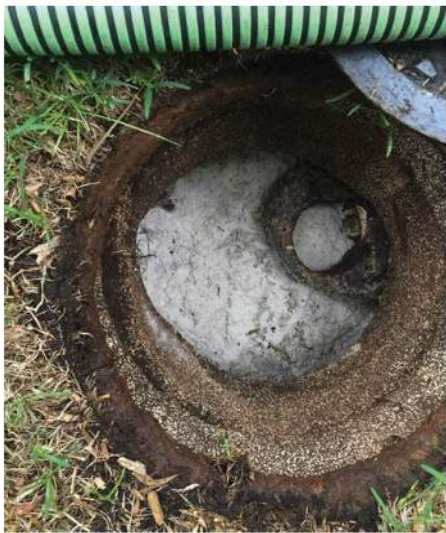
Proper maintenance and cleaning of grease interceptors is necessary because of the potential odors could become a public
